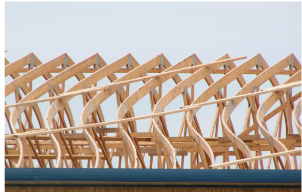
Trusses buckling during construction
